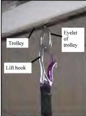
Figure 8B - Photo showing close-up of lift hook connected directly to eyelet of trolley.
